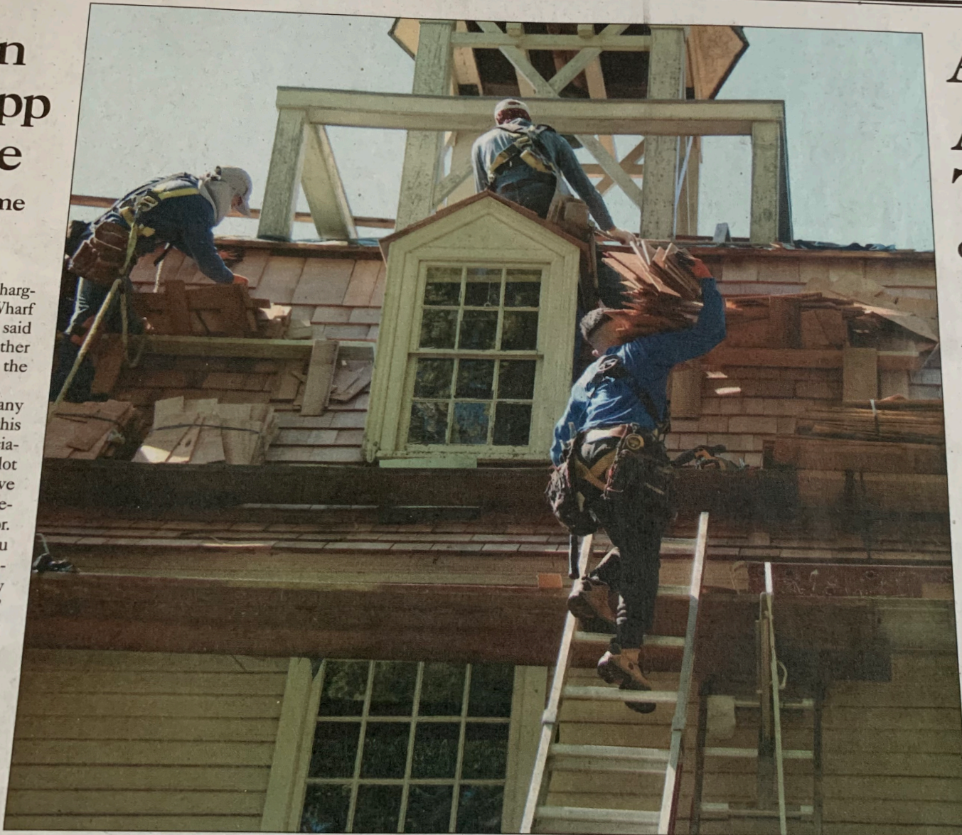
A fine balance. A crew was hard at work last week reshingling the roof of the East Hampton Historical Society's Clinton Academy.
