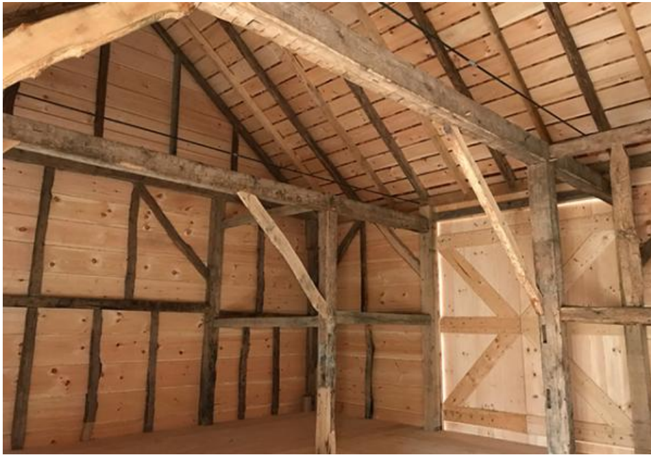
The interior view shows the combination of original, repaired, and new white oak framing. Mark Segal
